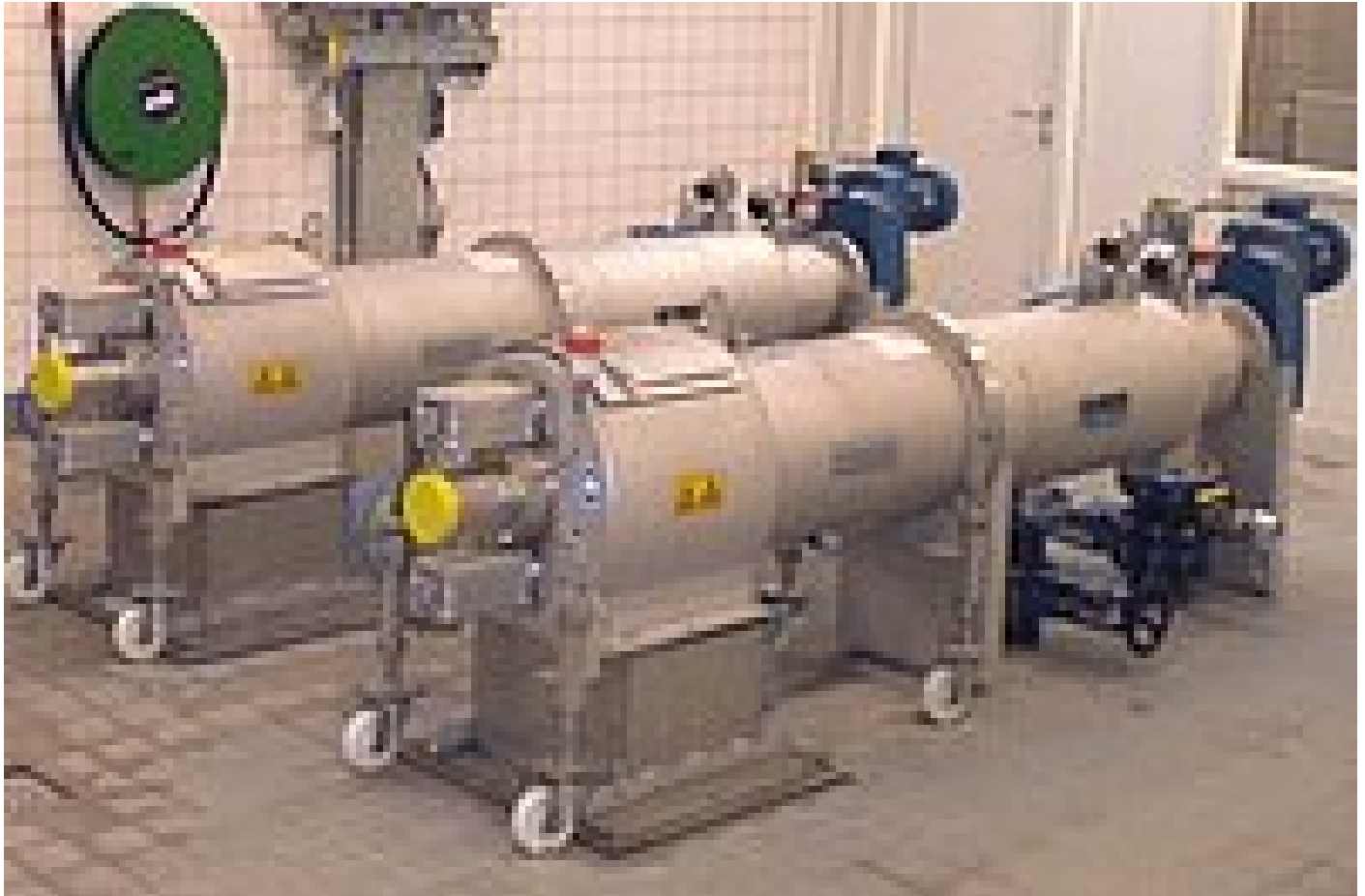
Two of the four STRAINPRESS® units installed on site
