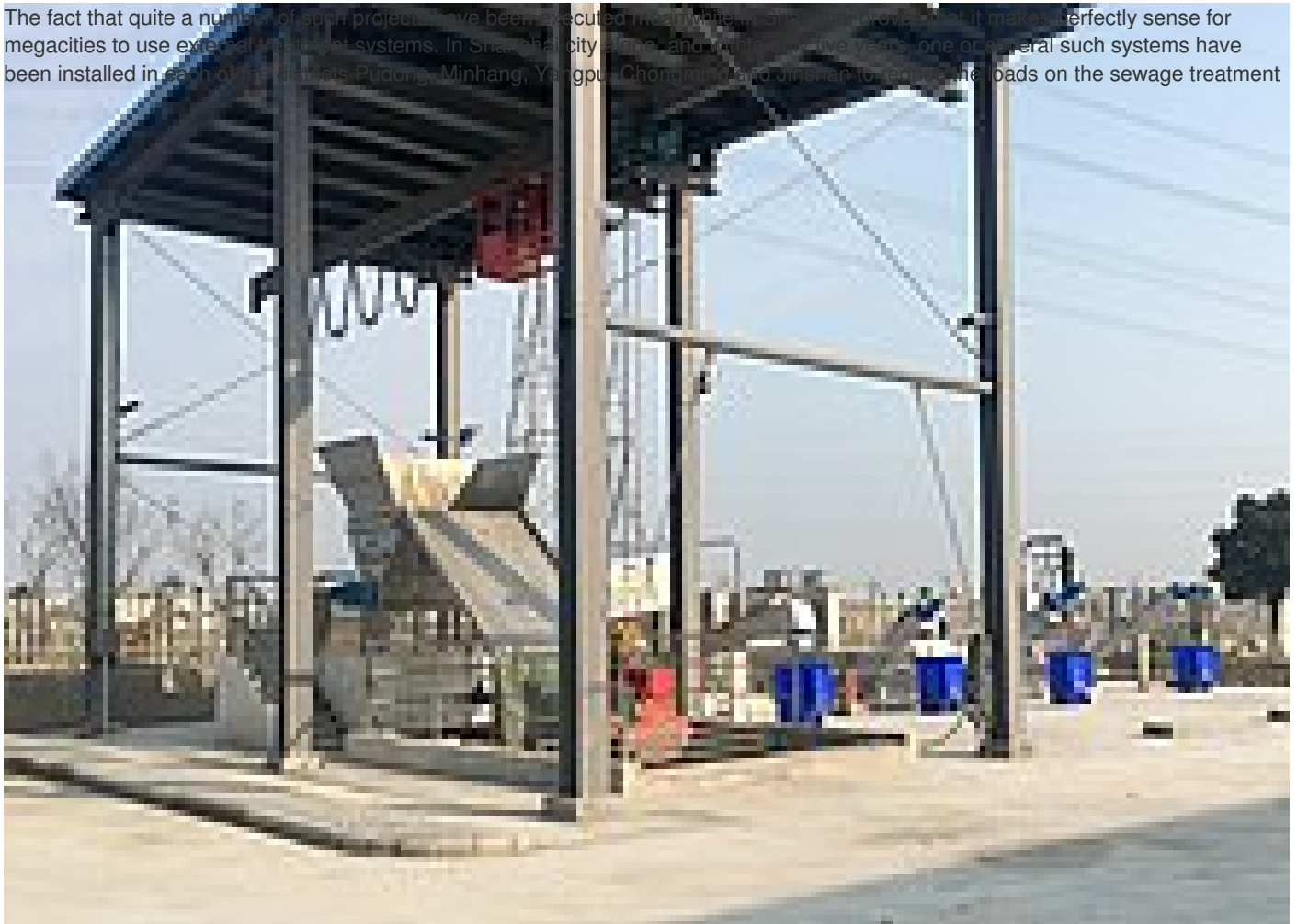
Fig. 2: Grit treatment plant in Kunshan, China
