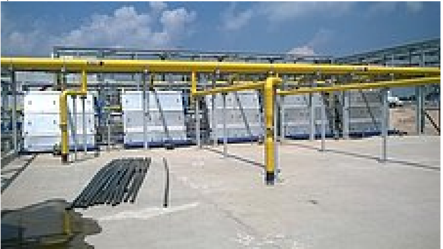
WWTP Atotonilco, the first of two coarse screen lines with 5 big HUBER RakeMax® screens, with direct discharge into a HUBER Launder Channel HLC with a length of 30m
