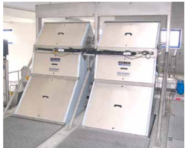
Two HUBER Fine Screen STEP SCREEN® SSF units installed in parallel channels.
